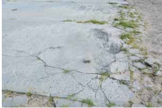
b) Weathered and cracked surface conditions and lack of proper cleaning and maintenance.
