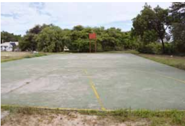
Faded line marking on Basketball court.
