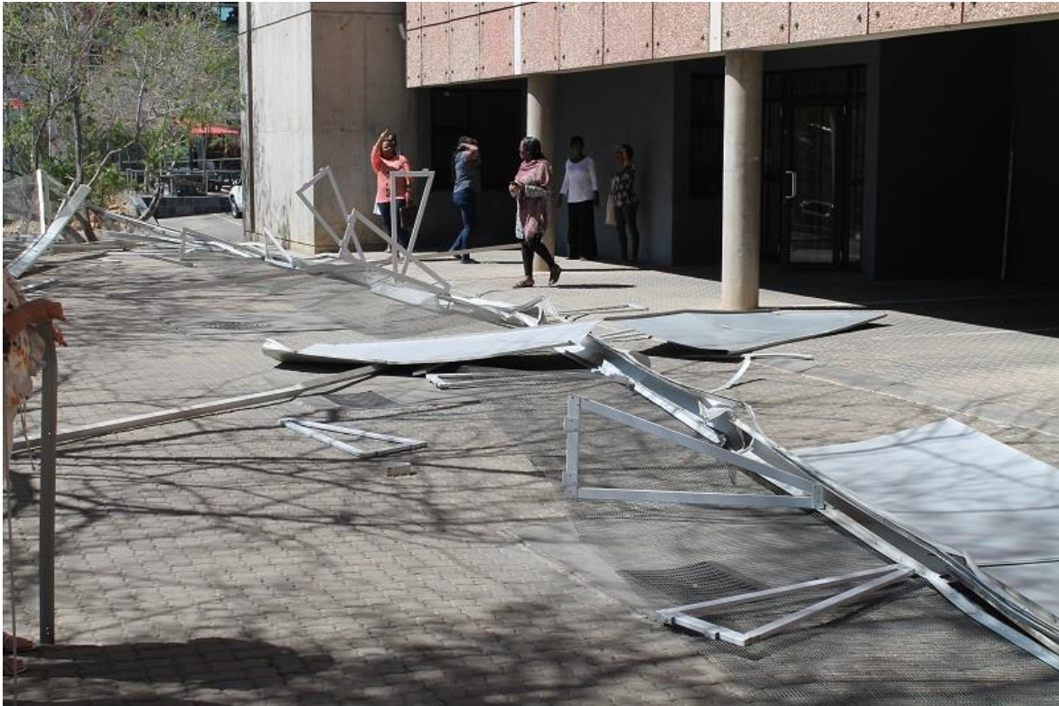
Part of the roofing material from the building that fell off late last year in 2017.
